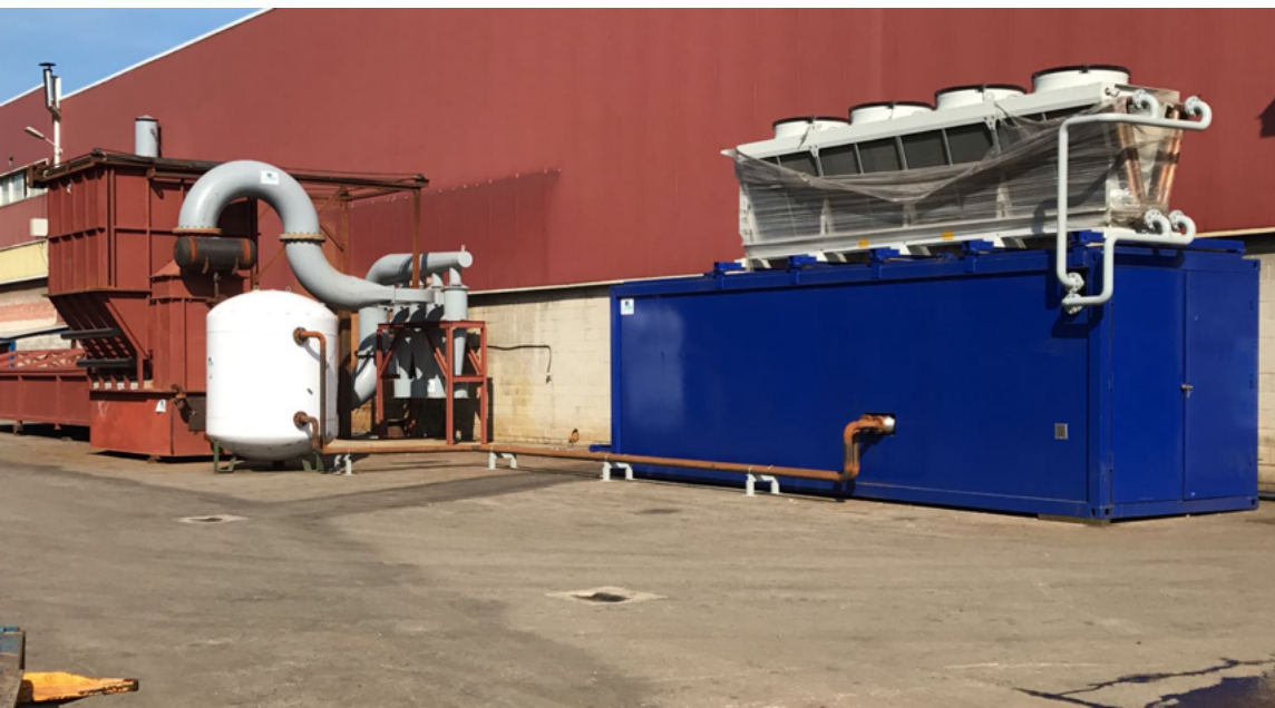
50 kW e ORC plant (courtesy of ENERBASQUE).
