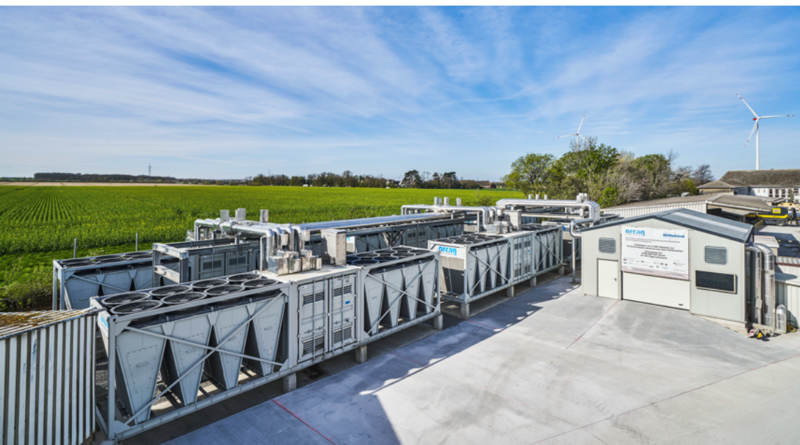
Heat recovery plant installed at the Wittekind cement plant. The ORC plant produces 8,000 MWh of electricity per year (courtesy of ORCAN).
