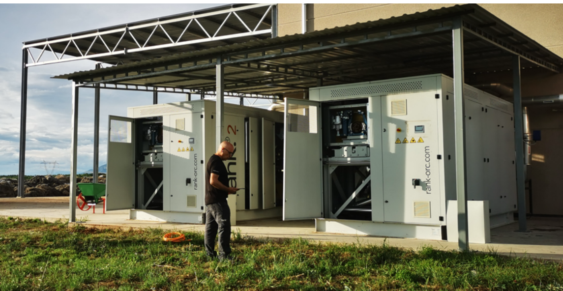
Two installed ORC units (courtesy of RANK).
