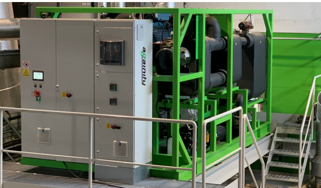
450 kW_e ORC power plant (courtesy of Againty).
