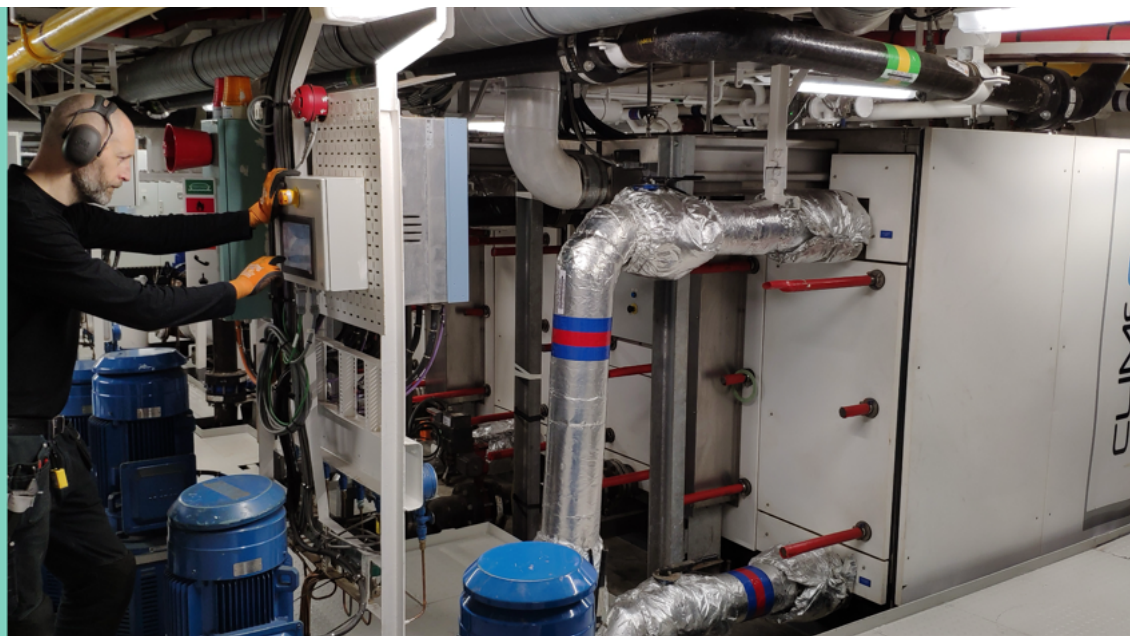
Heat recovery system installed on-board a shipping vessel (courtesy of Climeon).
