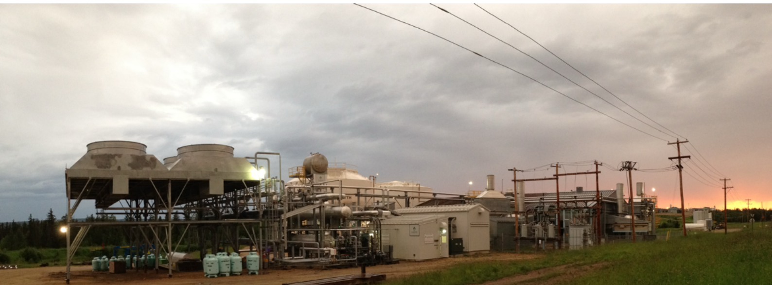
ORC power plant (courtesy of Atlas Copco).
