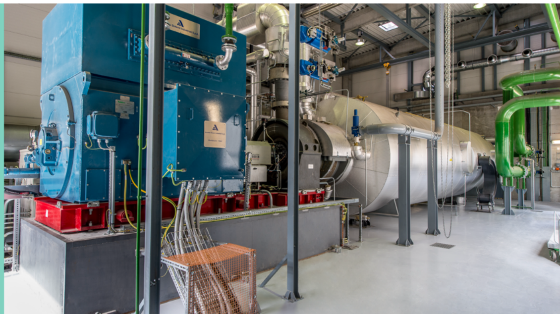
ORC power plant (courtesy of Turboden).
