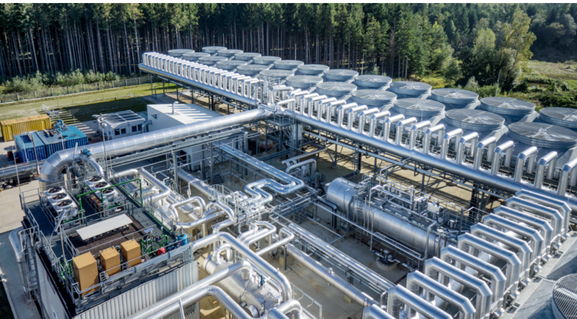
Large-scale ORC power plant (courtesy of Turboden).
