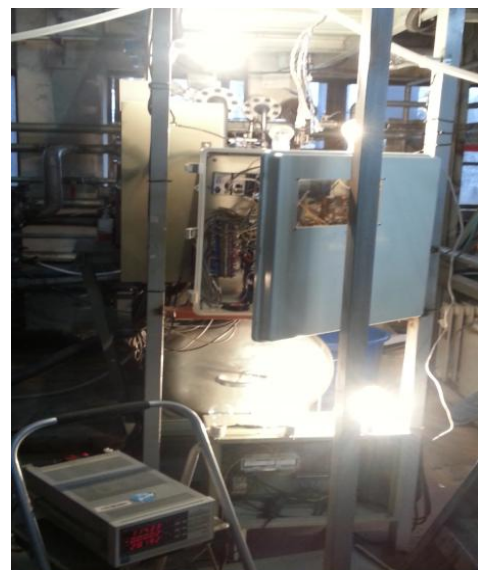
Figure 3: System under operation
